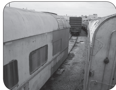
The Lounge-end of Diner 741 where the Maintenance of Way-installed doorway has been closed off.
